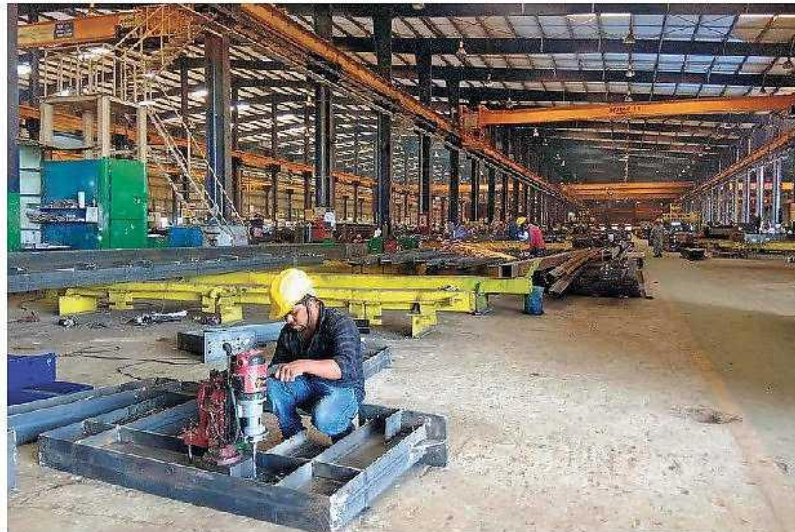
A worker making a steel structure at PEBS Pennar plant near Sadasivpet, about 75 km from the city. ■ N. RAVI KUMAR
